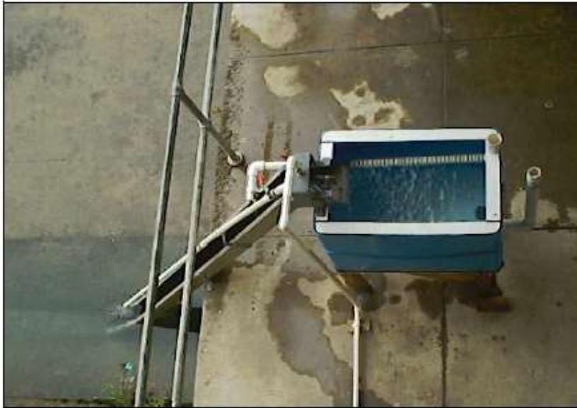
Figure 17: Example of trap installation at dam.
