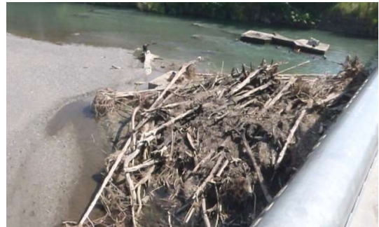
8D. Accumulation of wood at the bridge pile
