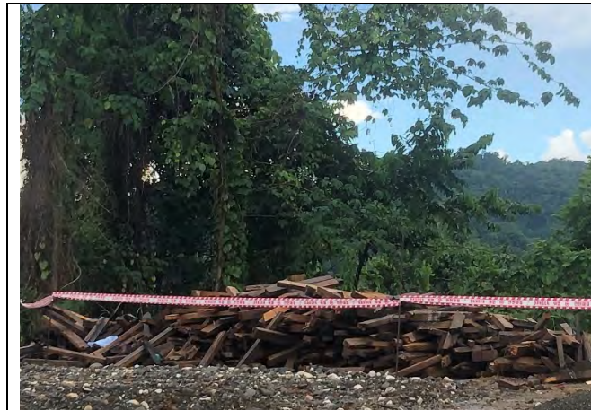
Figure 3-3: Danger tape being used on site, November 2022
